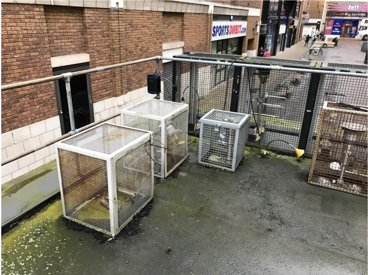
Figure 3-7 ZAURN Co-Location Z787 & 799
